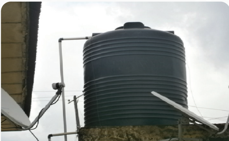
Water supply at Maikunkele PHC refurbished, new storage tank installed, borehole drilled by community stakeholders
