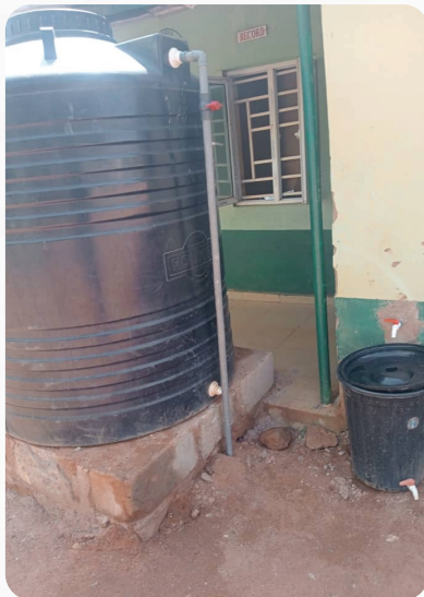
Water installation at Pindiga PHCC
