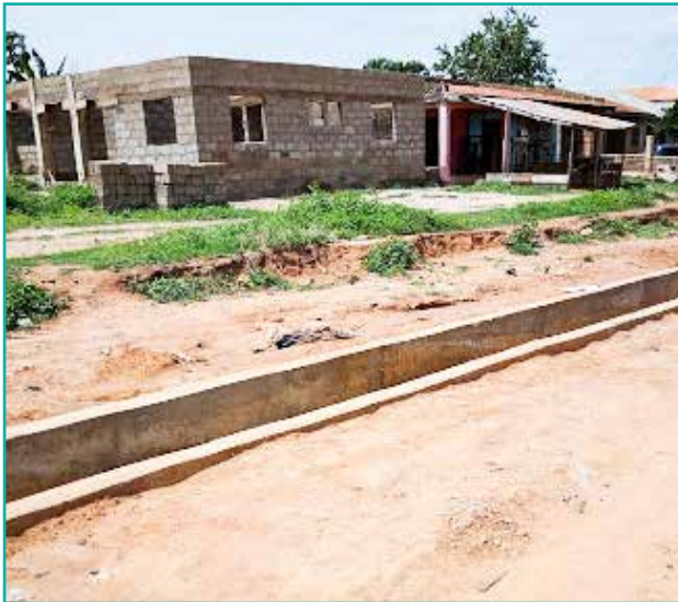
Drainages Construction, Road Improvement, and Erosion Control at Kilanko-Elegbede-Micheal Imodu, Ilorin South LGA, Kwara State
