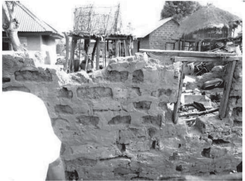
Affected building in Ijiwo Village, Akpe LGA
