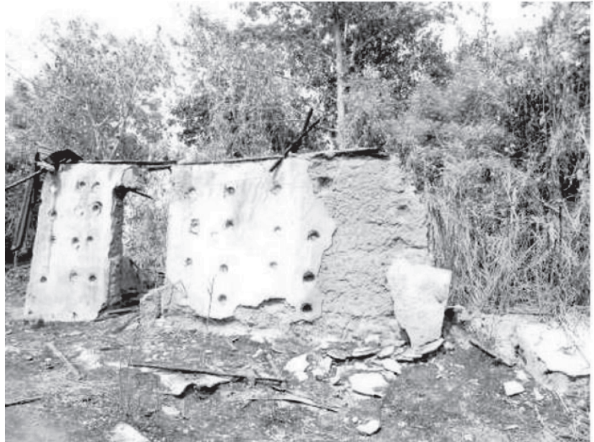
A community destroyed by flood in Chewuru
