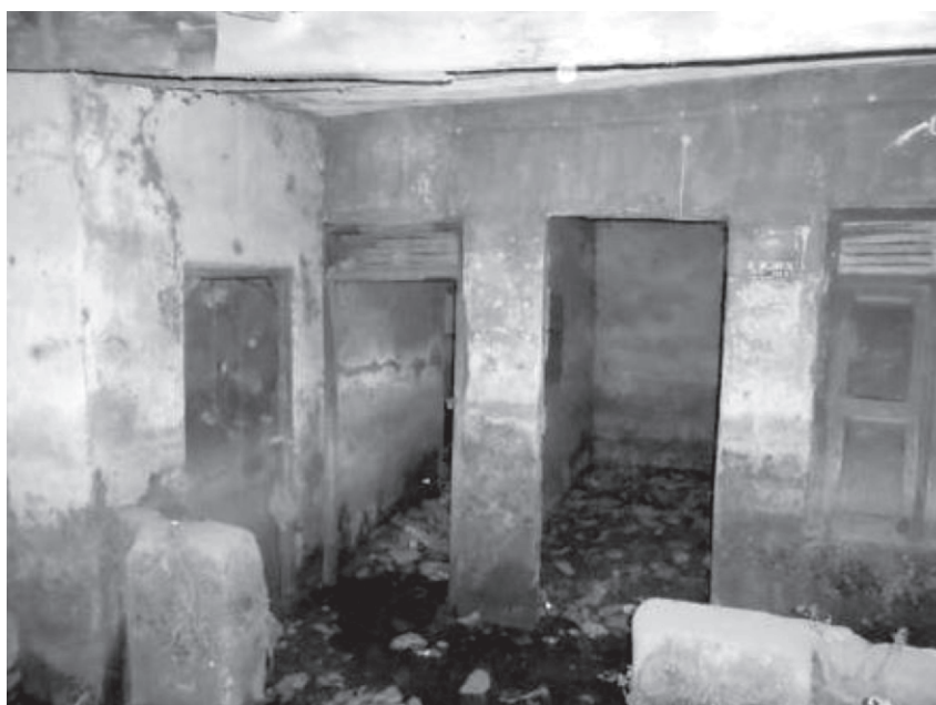
An abandoned building destroyed by flood in Onyemadi Road, Abia State
