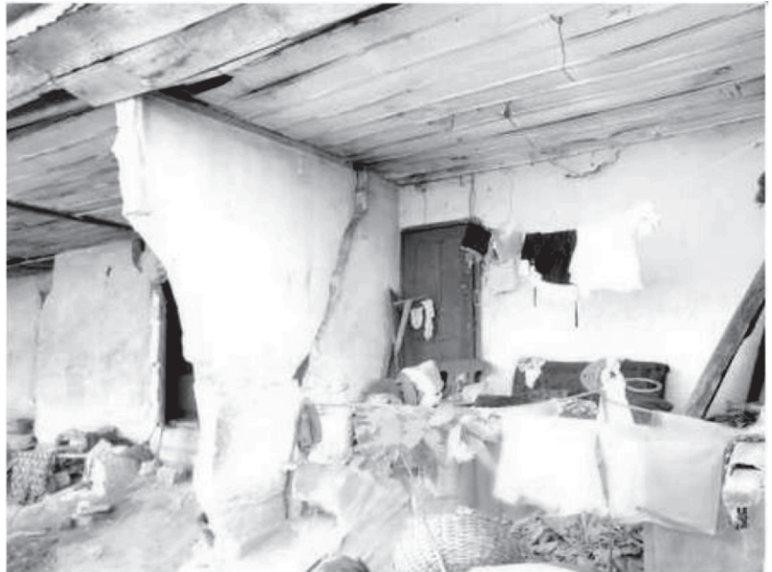
One of the Affected building in Oguta Community
