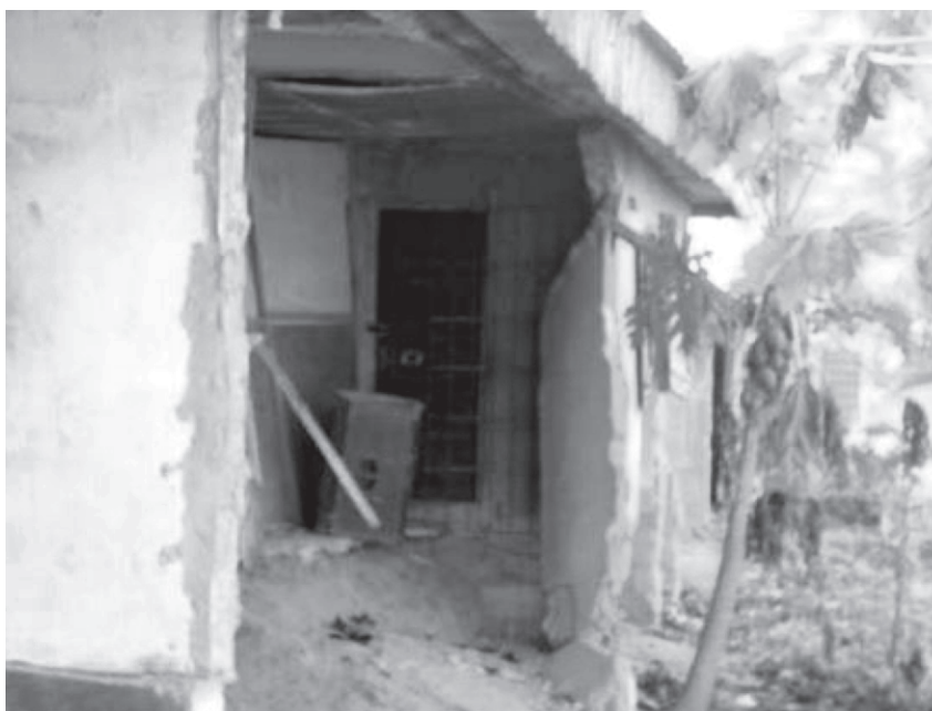
One of the Affected building in Oguta Community
