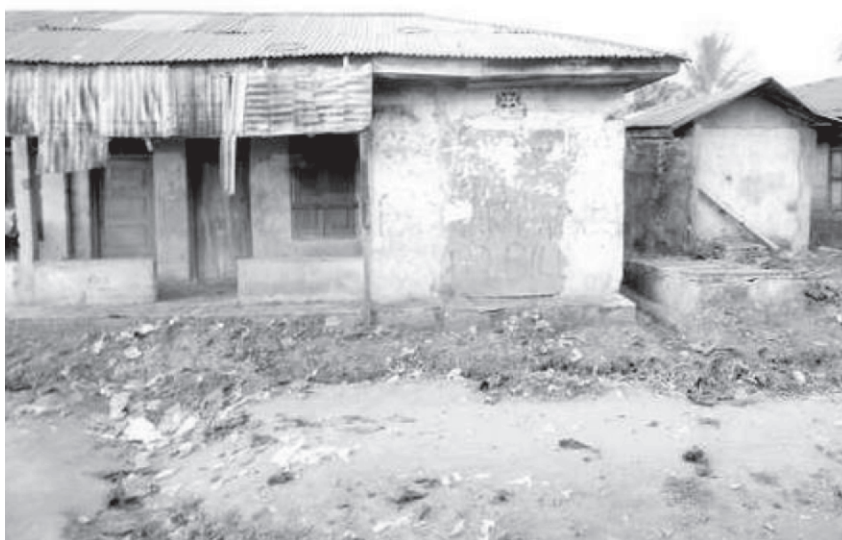
An abandoned building destroyed by flood in Ohanku Road, Abia State
