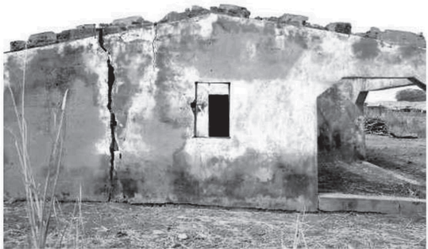
The Clinic submerged by Flood in Ketso, Mokwa LGA
