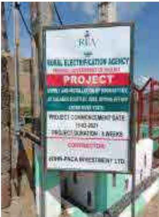
Procurement and Installation of 300 KVA Transformer at Effiong Effiom Close, off Jeb Road, Calabar South LGA
