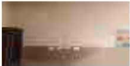
A section of the walls structure implicated by the rain from the leaky roof.
