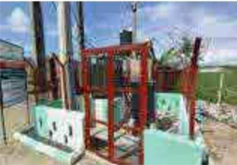
Procurement and Installation Of 300kva Transformer at Effiong Effiom Close, Off Jeb Road, Calabar South LGA
