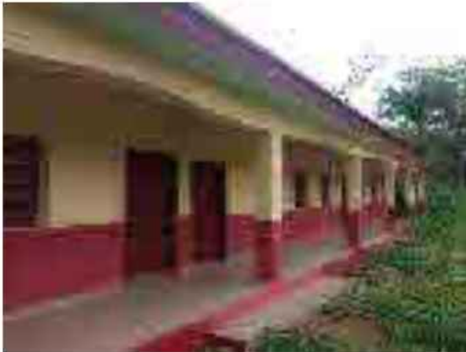
Construction of 1 No.6 Class Rooms Block for Modern Primary School Amansiodo Oghe, Ezeagu LGA, Enugu State.
