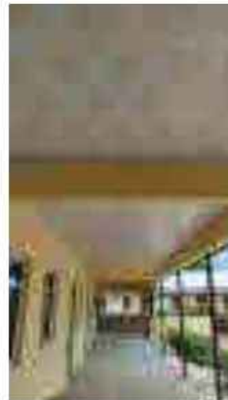
Renovation of Health Centre in Okrika Nweke, Akpim, Ahiazu Mbaise, Imo State
