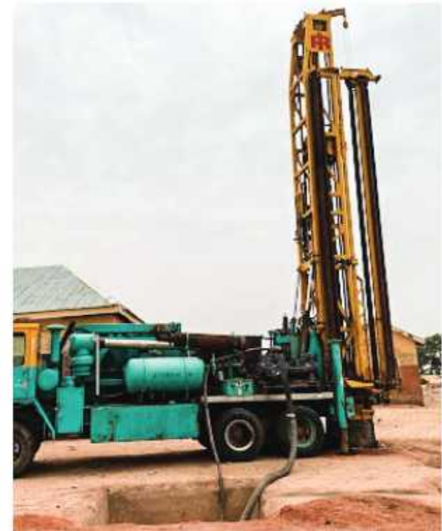
Shongo, Sarkin Yaki stalled water project (Amount: N50m)
