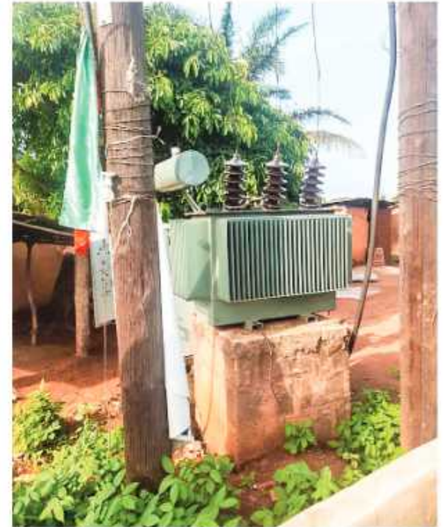
Supplied transformer to some communities in Otukpo/Ohimini Federal Constituency, Benue State (Amount: N15m)
