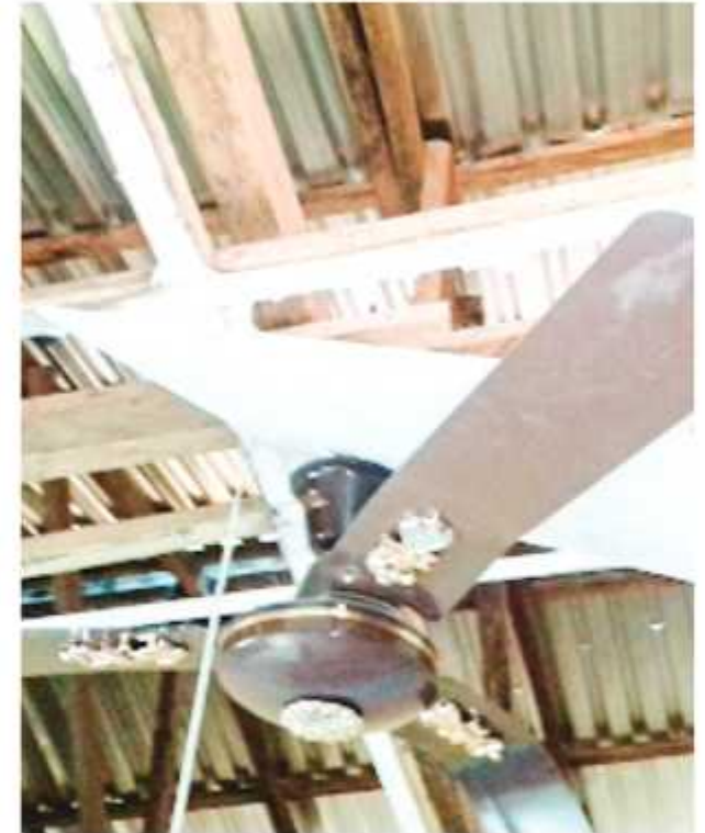
Barely six months after renovation, rooftop of Agu Ugwu Health Centre was destroyed (Amount: N40m)
