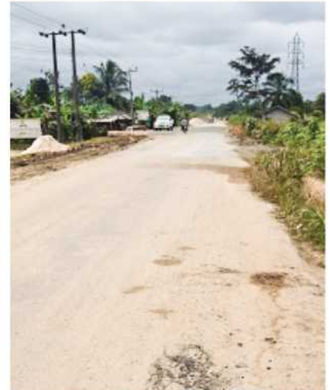
Repair Of Ahoada-Abua-Degema Road, Rivers West Senatorial District, Rivers State (Amount: N100m).
