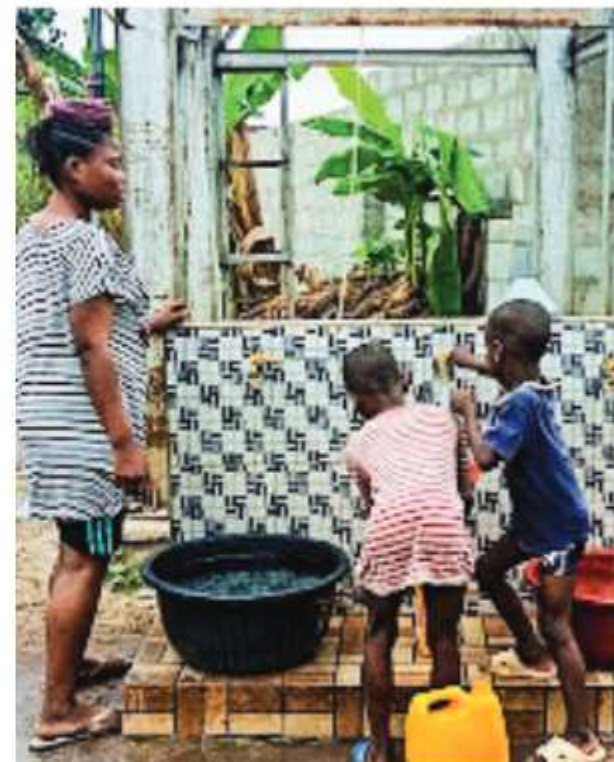
Solar-powered borehole serving Agbala community, Owerri North LGA, Imo state (Amount: N13.5m)
