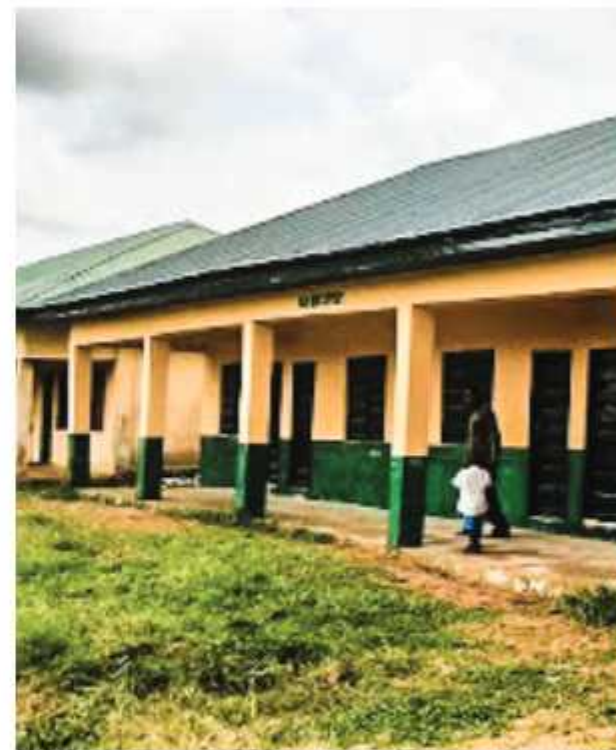
Completed but unused classrooms in Methodist Primary School, Oruko, Urue Ofong LGA (Amount: N20m)
