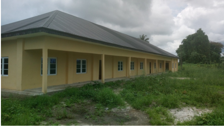
COMPLETION CONSTRUCTION OF NDON TOWN COMMUNITY HALL NDON MPAT ENIN LGA AKWA IBOM STATE
