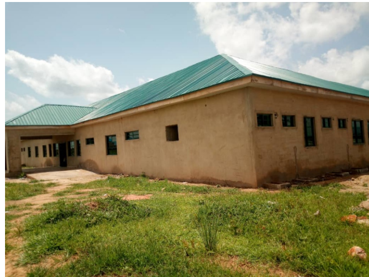
CONSTRUCTION OF COTTAGE HOSPITAL AND SUPPLY OF MODERN MEDICAL EQUIPMENTS AT DADIN KOWA, DOGUWA LOCAL GOVERNMENT, KANO STATE.
