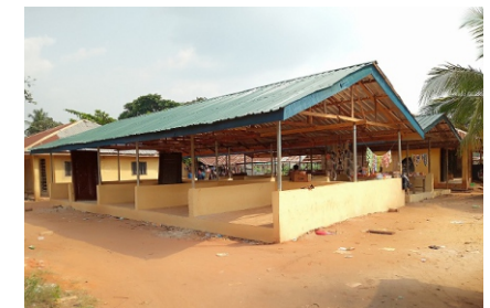
REHABILITATION OF EKE-UKWU LORJI MARKET IN ABOH MBAISE LGA OF IMO STATE (3)
