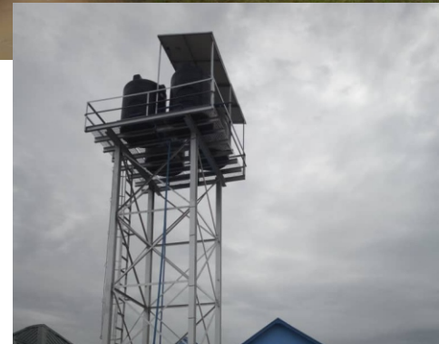
DRILLING OF BOREHOLE AND INSTALLATION OF 100,000 LITRES CAPACITY TANK WITH SOLAR AT OPOLO-EPIE HEALTH CENTER IN BAYELSA CENTRAL SENATORIAL DISTRICT, BAYELSA STATE.
