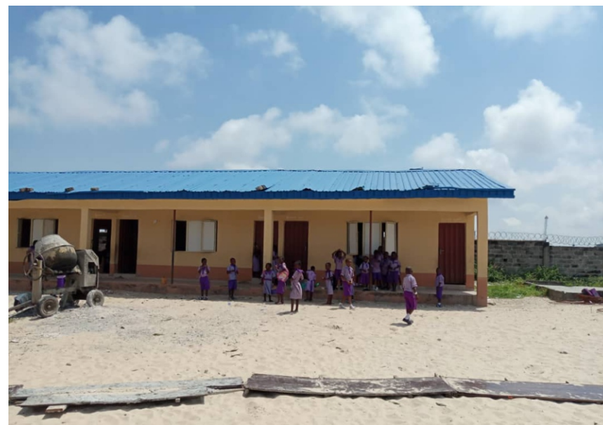
PROVISION OF TOILET FACILITIES WITH MOTORIZED BOREHOLES IN TWENTY PRIMARY AND SECONDARY SCHOOLS WITHIN LAGOS CENTRAL SENATORIAL DISTRICT.
