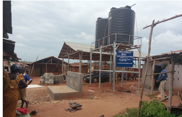
CONSTRUCTION OF MOTORISED BOREHOLE AT AJEBANDELE IJEBU EAST LG, OGUN EAST SENATORIAL DISTRICT, OGUN STATE.
