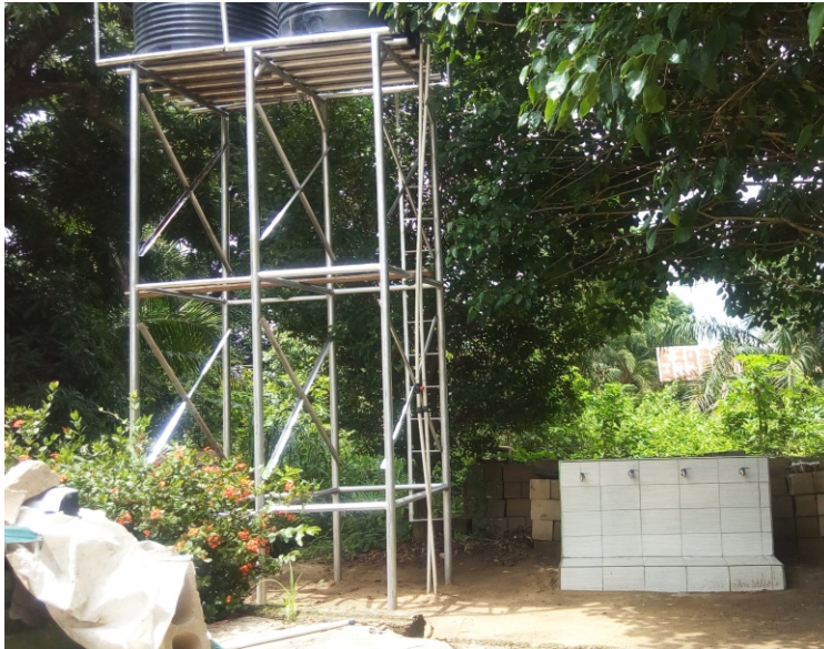
PROVISION OF 6 NO'S MOTORIZED BOREHOLES WITH GENERATOR AT IDAH,IGALAMELA-ODOLU, OFU AND IBAJI FEDERAL CONSTITUENCY KOGI STATE
