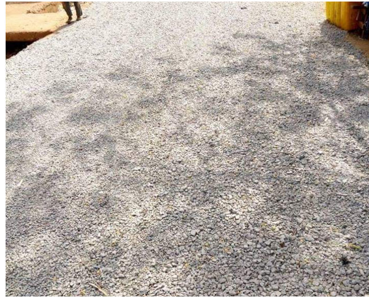
TARRING OF ROAD IN ACHIDA TASHA-JUNCTION TO KWASARE PRIMARY SCHOOL, WURNO LGA, SOKOTO STATE.
