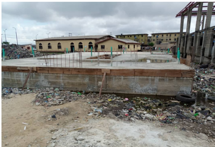
CONSTRUCTION OF PRIMARY HEALTH CENTER TYPE B WITH SOLAR POWER AND FENCING AT LUTHER STREET, LAGOS ISLANDII FEDERAL CONSTITUENCY
